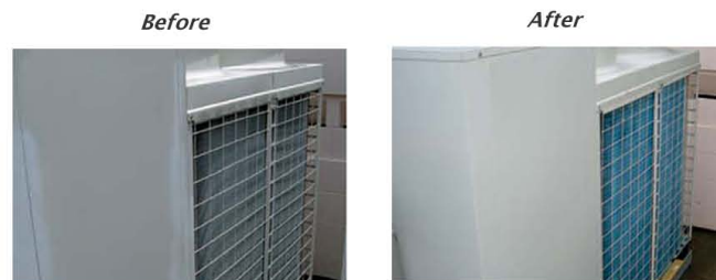
Condensing units Before and After AerisGuard Maintenance
